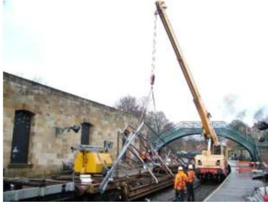
Construction of the new overall station roof utilising materials brought to site by rail
